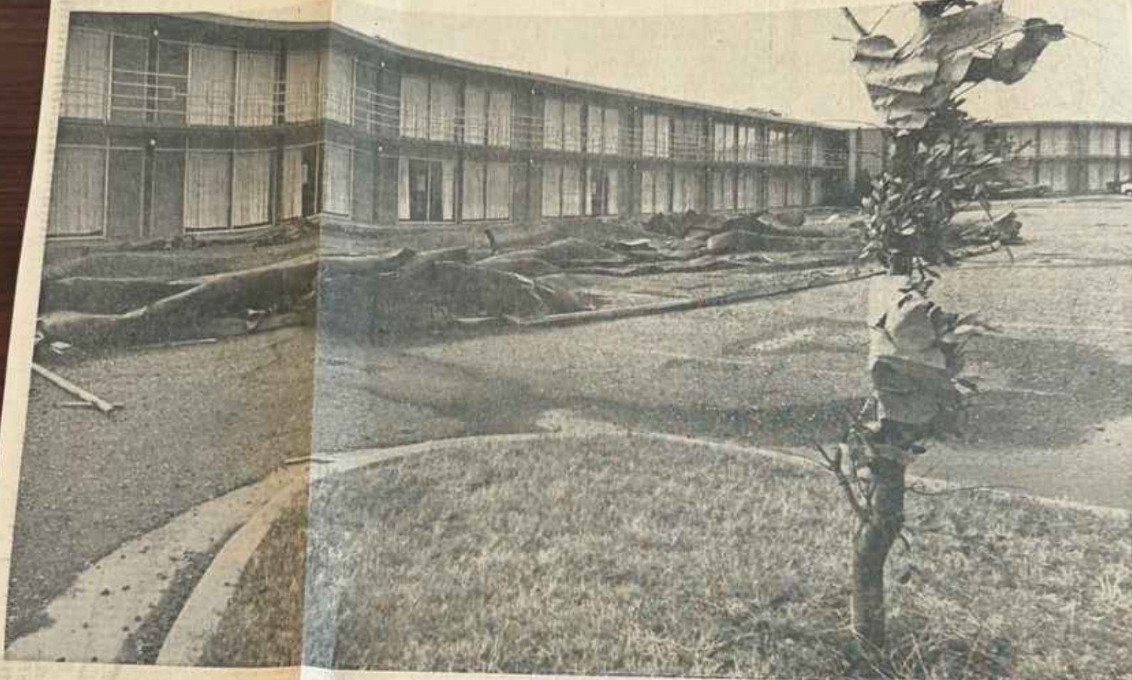
Twisted sections of roof blown from the Quality Courts Motel on Willoughby Spit lie in the parking lot.
